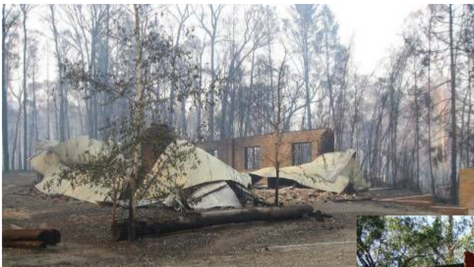
Above: SouthWest view of the destroyed Kitchen / Dining room
